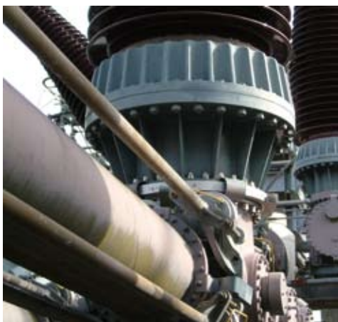
Typical SF 6 Filled Substation Equipment
