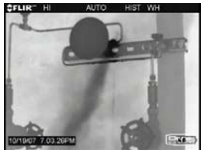
A leaking pressure gauge
